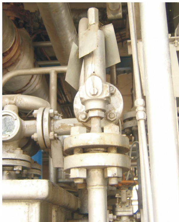
Pressure Relief Valve in Hard Alloy Mill
