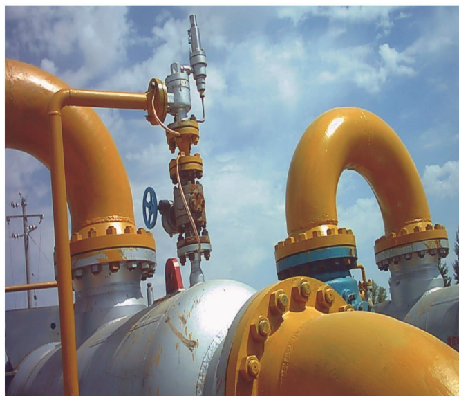
Pilot Safety Valve in Gas Field
