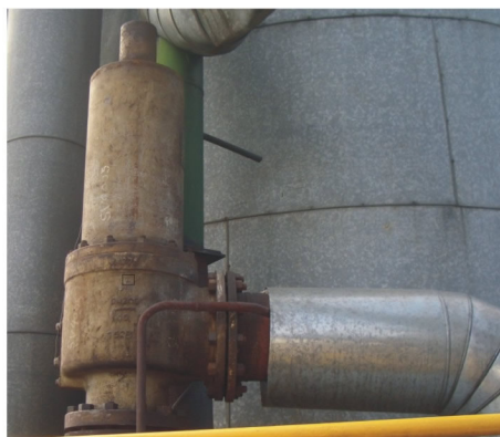
Coventional Safety Valve in Textile Factory
